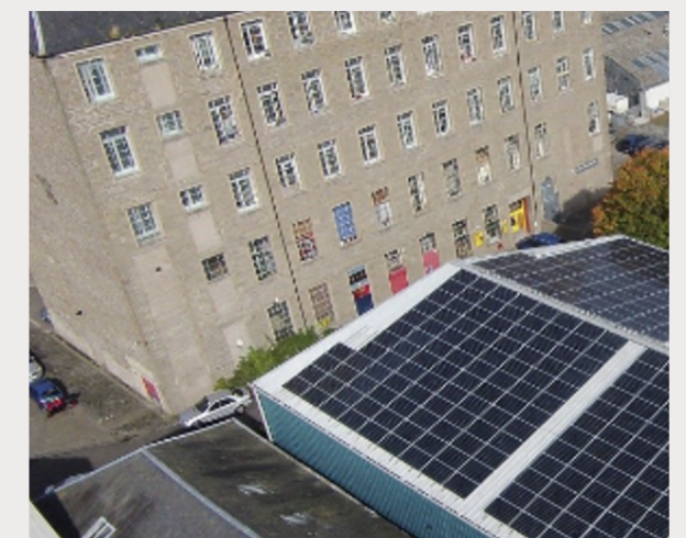
Dundee Industrial Association's (DIA) solar photovoltaic arrays (2 x 50 kW) opposite Wasps' Meadow Mill building. Wasps pay a contribution to use 50kWp of solar energy to electrically heat the building.
